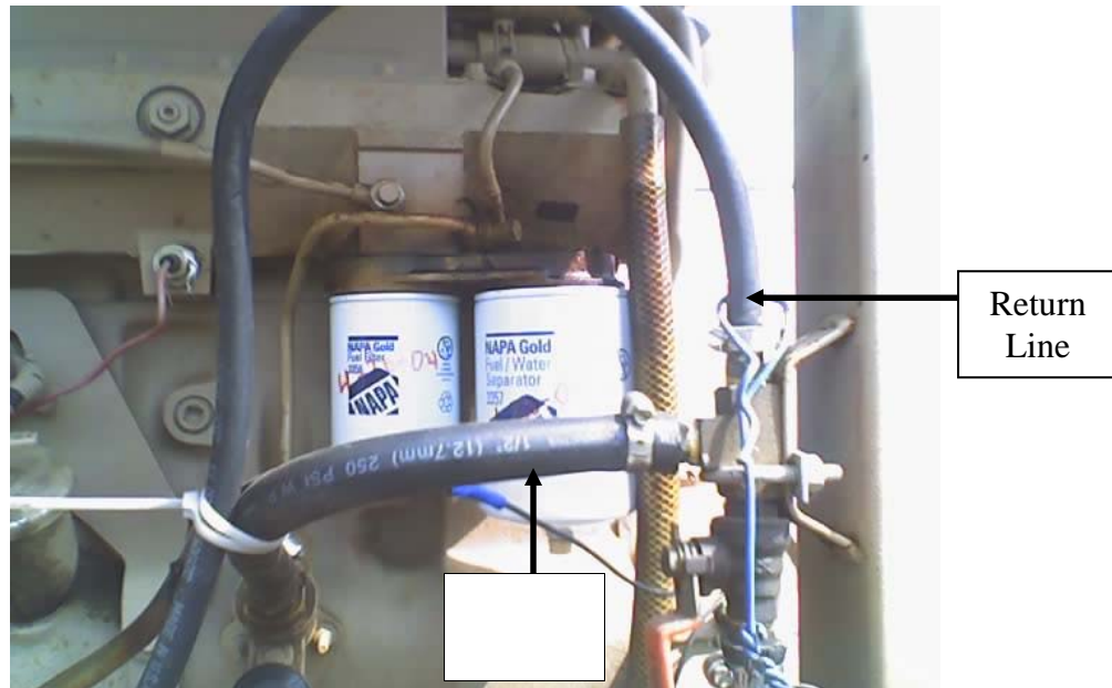
Figure 3, This engine has the return line and supply line looped at the engine. Not recommended by the engine manufacturer as there is not adequate cooling of the fuel before returning to the injectors.
