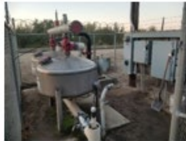
Pump & Filter Station
