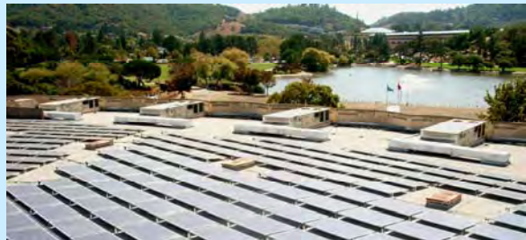
Solar panels line the rooftops at the Marin County Fair & Exposition in San Rafael
