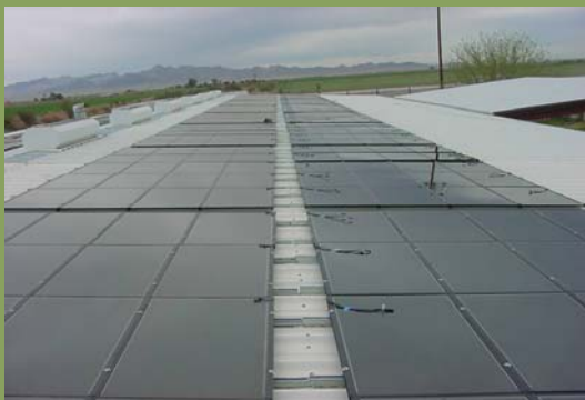
Solar panels line the rooftops at the Colorado River Fair in Blythe.
