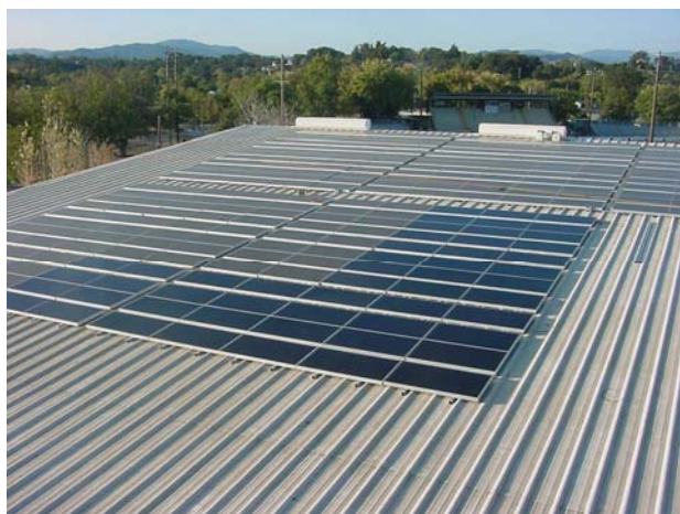
Solar panels line the rooftops at the Lake County Fair in Lakeport.
