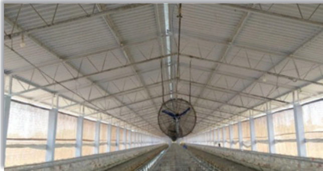
Fans increase air velocity and create a cooling effect.
