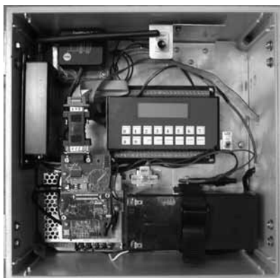
Figure 3 a, b Third generation wireless valve controller and field controller.
