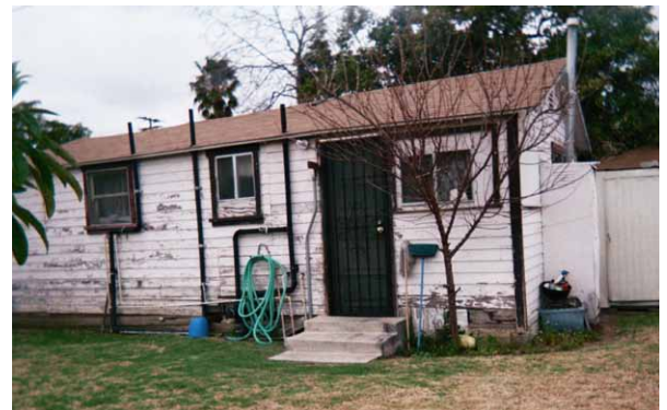
Existing farmworker housing in need of repair. Photo courtesy of Cabrillo Economic Development Corporation.
