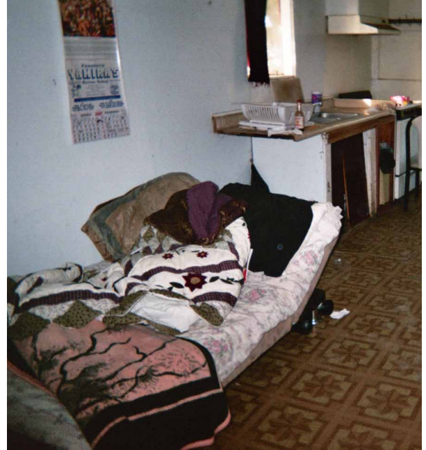
Existing farmworker housing in need of repair. Photo courtesy of Cabrillo Economic Development Corporation.
